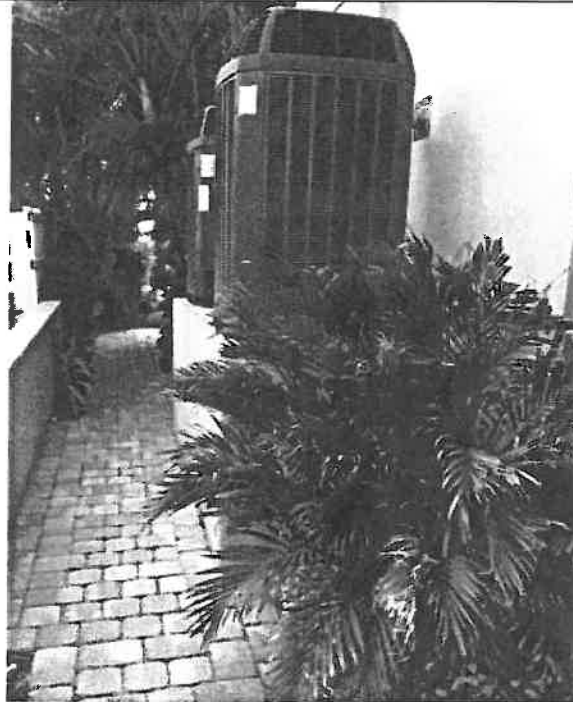
Photo One Caption Photo Taken 2/22/2018 "Side View With A/C Pad"
